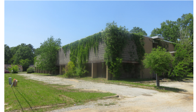
Blighted property at corner of Augusta Ave. & Norman Bridge Rd.
